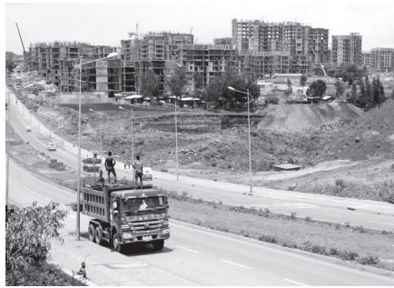
Chefie housing estate at the eastern periphery of Addis Ababa, Ethiopia. Part of one of the largest ongoing social housing initiatives on the African continent. Courtesy C. Marcinkoski.
